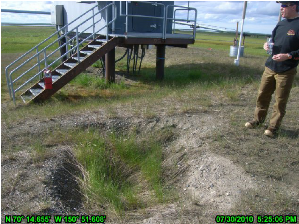
PHOTO A.5 HDD WEST, JULY 30, 2010: PIT IN GRAVEL PAD EAST OF CP MODULE BUILDINGS
