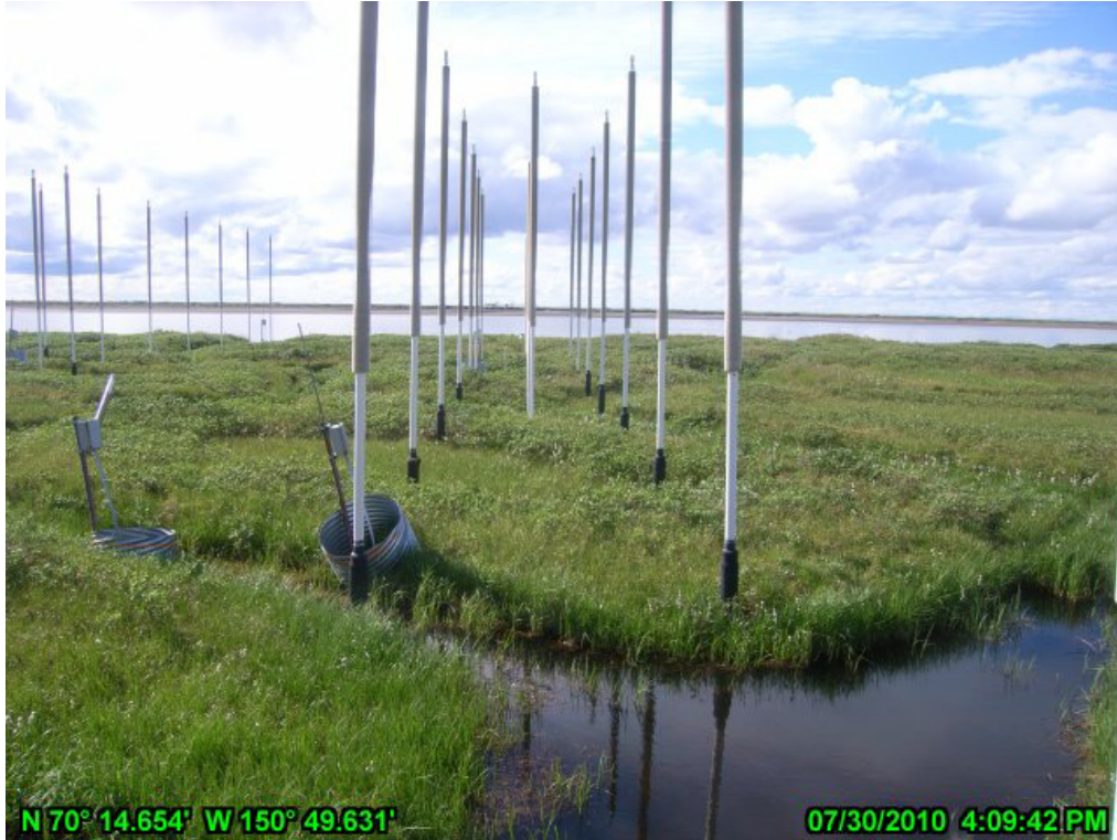
PHOTO A.13 HDD EAST, JULY 30, 2010: LOOKING WEST THROUGH THERMOSIPHONS WITH TROUGH IN FOREGROUND
