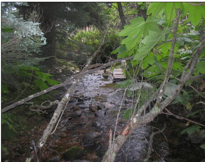
Narrow mixed control channel (MM1). View looking downstream toward culvert inlets and Dyea Road. Image: A. Bethe, TIWC, August 2005.
