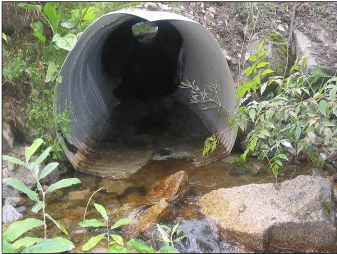
One of two culverts under Dyea Road at Matthews Creek. Note the steep grade. These culverts likely present a sediment transport and fish passage problem. Image: A. Bethe, TIWC, August 2005.
