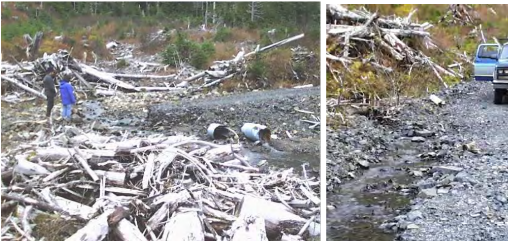
Photo 23. Relief culvert plugged and subsequent stream crossing failure. Photo 24. Relief culvert failure.
