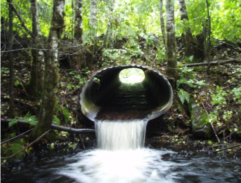
Photo 5. Culvert crossing on Road 6308 is likely juvenile fish barrier.
