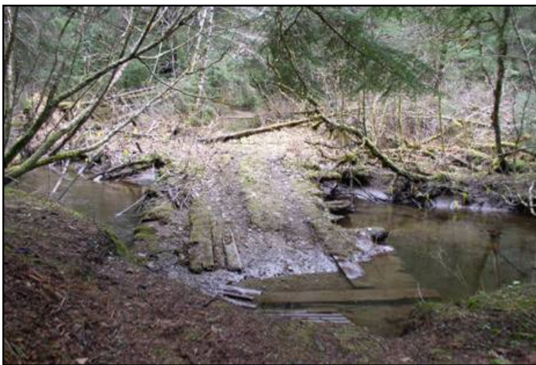
Figure 13: Collapsed bridge near Sasha Street. April, 2005.
