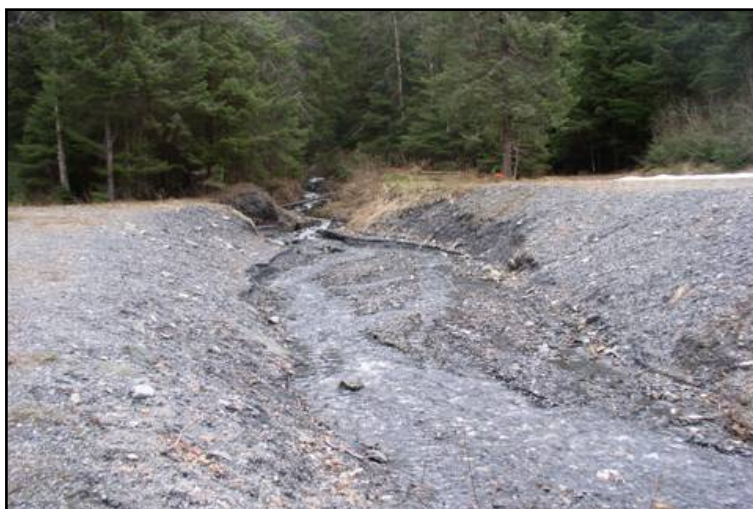
Figure 7: Streambank erosion near the City water tower. The tower is located to the right of the stream. April, 2005.
