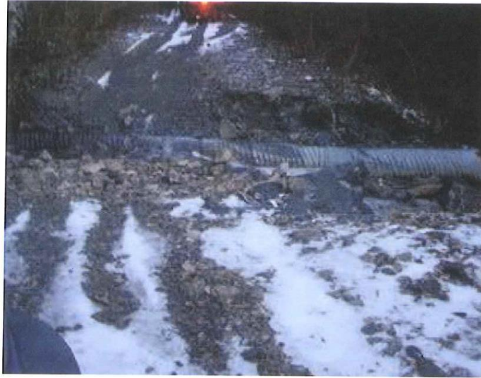
Figure 12. Failed culverts on Dog Salmon Creek may block passage.
