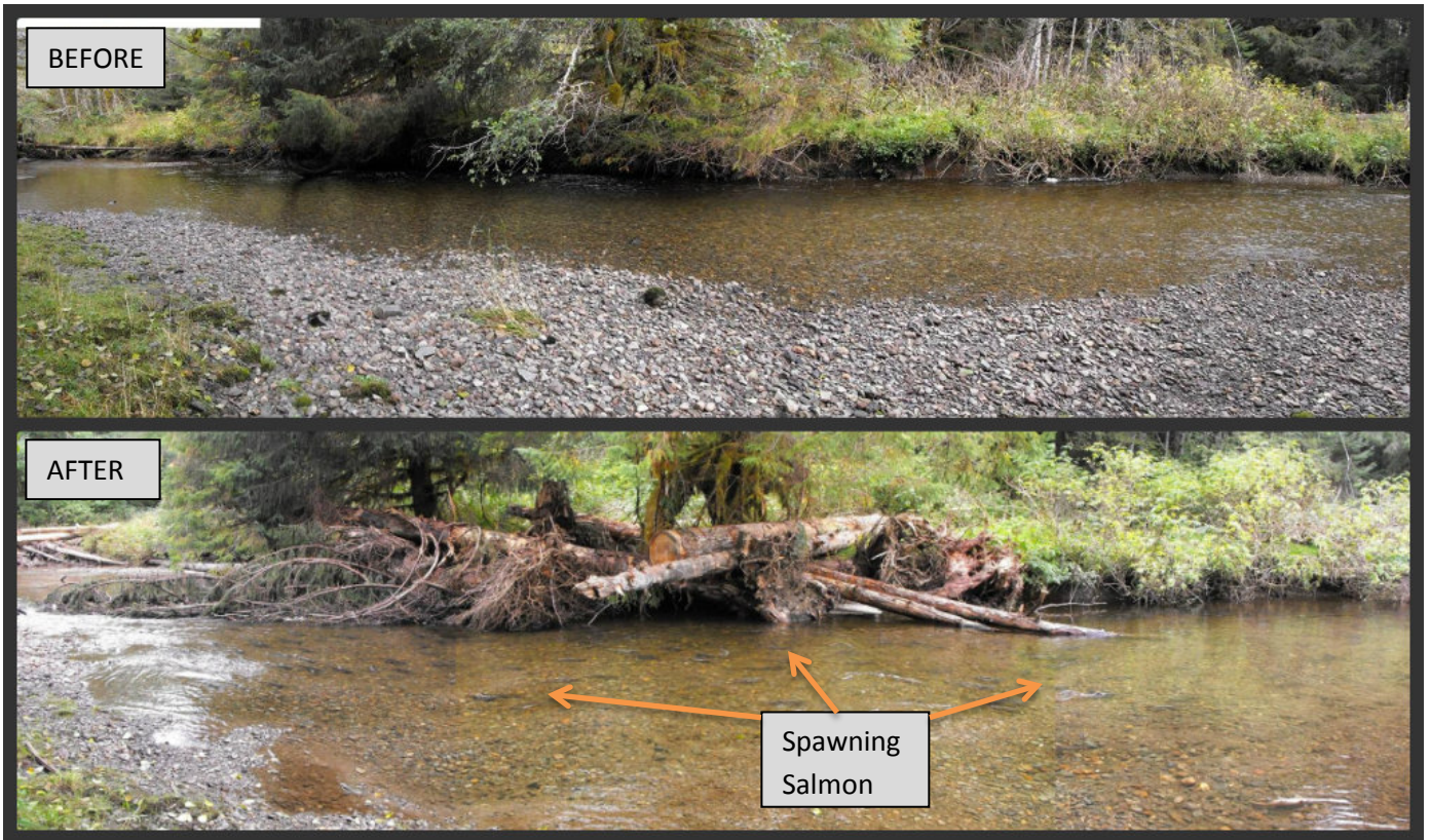
Photo set 2 – Phase II, Structure Number 16.5, looking downstream right bank before and after LW placement.
