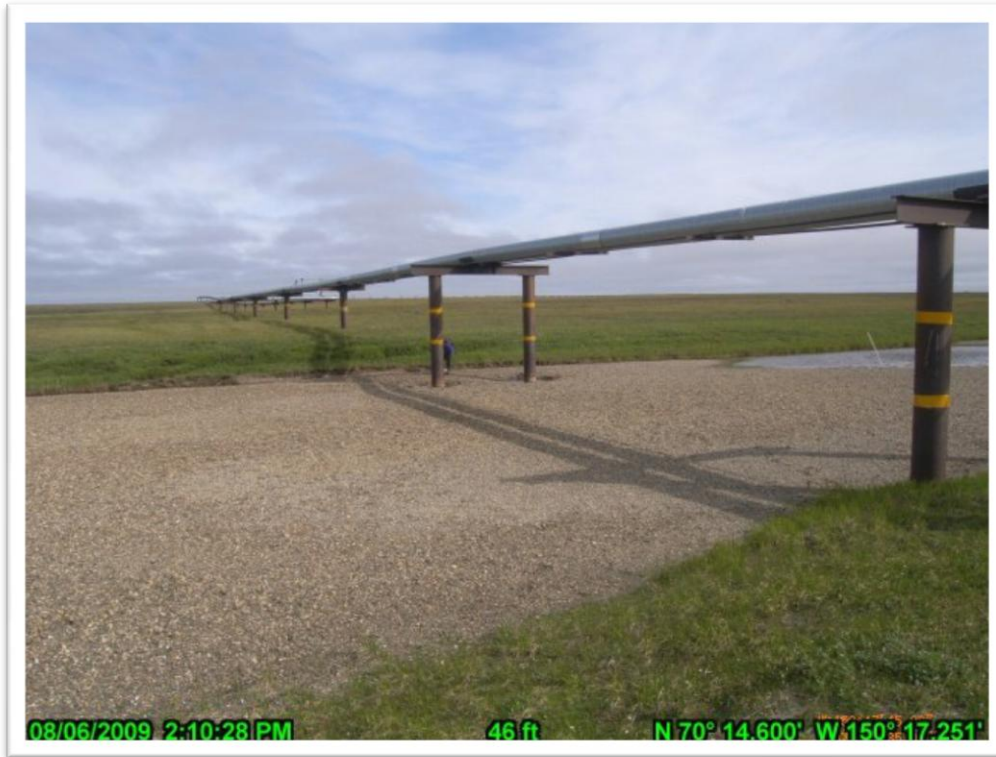
PHOTO A.29 MILUVEACH RIVER CROSSING, AUGUST 6, 2009. VIEW OF EAST BANK LOOKING SOUTHEAST.
