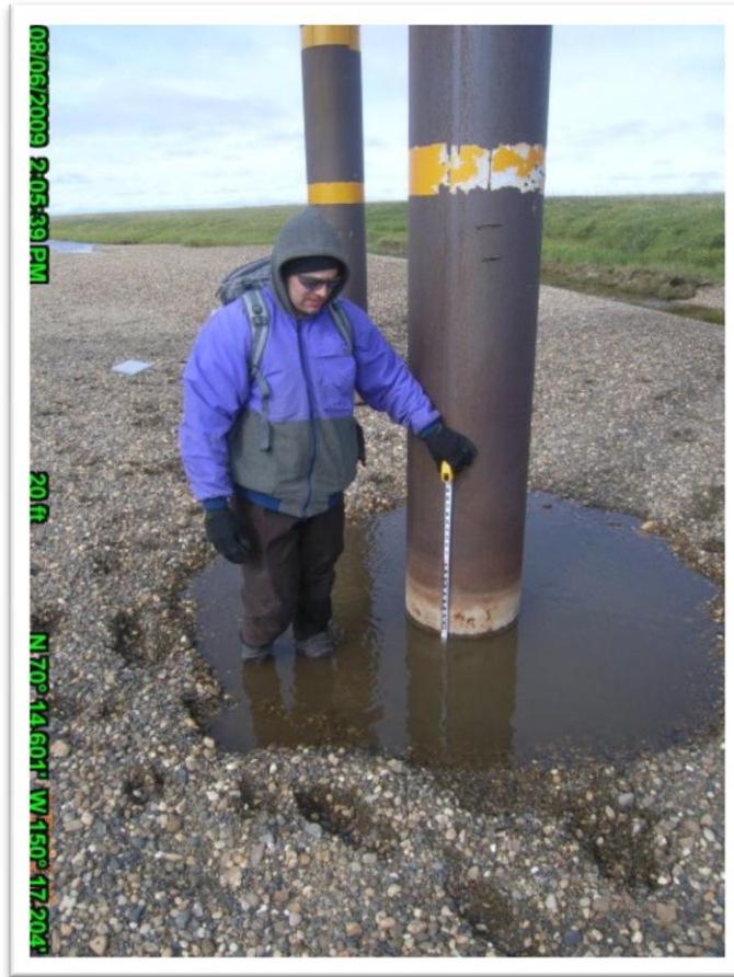
PHOTO A.27 MILUVEACH RIVER CROSSING, AUGUST 6, 2009. VIEW OF VSM SCOUR HOLE.
