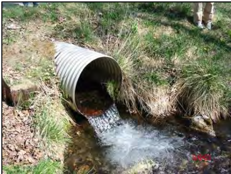
Figure 9: Perched culverts like this one create formidable and sometimes impassable barriers to juvenile salmonids
