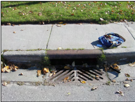
Figure 25: Stormwater catchbasins dot the town of Skagway
