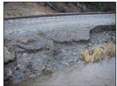
Figure 27: Sluffing of stream banks, as has occurred at this location along Pullen Creek, damages stream habitat and infrastructure necessary for community functions
