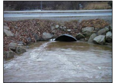
Figure 26: Culverts that are too small inhibit fish passage by increasing stream velocities, at negatively impact stream hydrology
