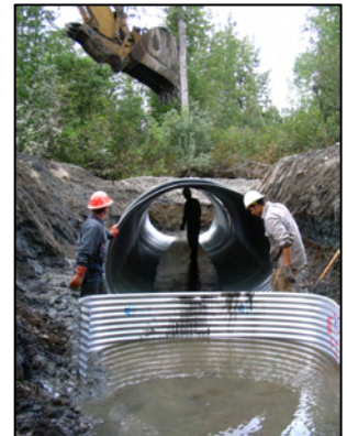
Figure 17: Replacing culverts which block fish passage is essential to restoring habitat and hydrologic function
