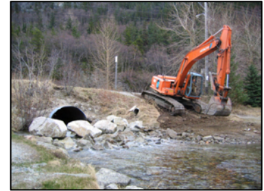
Figure 20: ADOT&PF installed this rock weir at the upstream end of Pullen Pond
