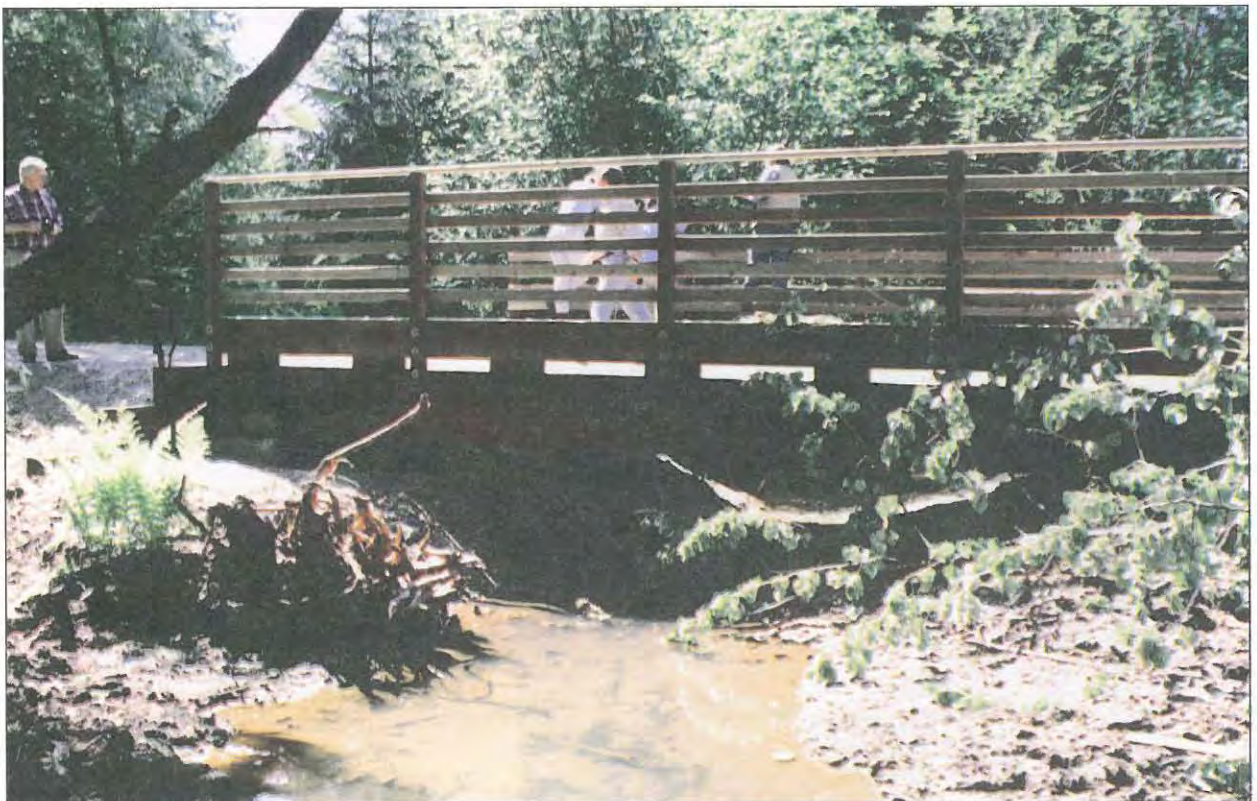
Figure 9.--Timber bridge used to replace a perched culvert on a private driveway. (Photo by NMFS).
