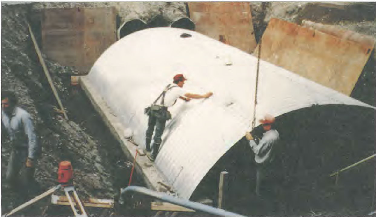
Figure 7.--Perched culverts being replaced with an arch culvert at Stephen-Richards Drive. (Photo by Jan Caulfield, CBJ).
