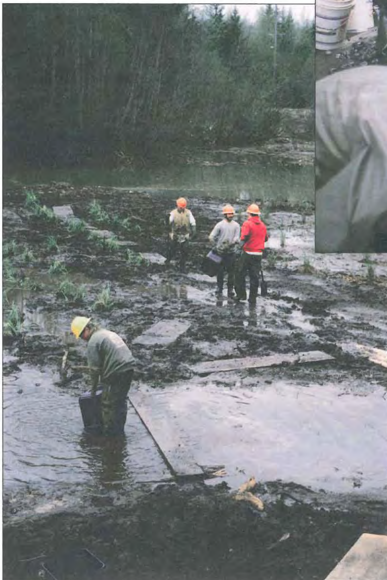
Figure 11.--Development of a stormwater treatment marsh in a dredge pond on the east fork of Duck Creek. (Photo by NMFS).
