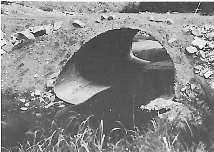
Figure 24.--Culverts which are placed directly on the original streambed, and where possible, made to conform with the streambed, create the best fish passage.
