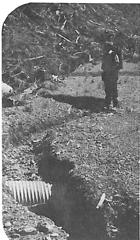
Figure 22.--Culverts which are not removed from abandoned roads, or maintained when left in, can become clogged. This could change stream channels, cause erosion, or block migrating fish.
