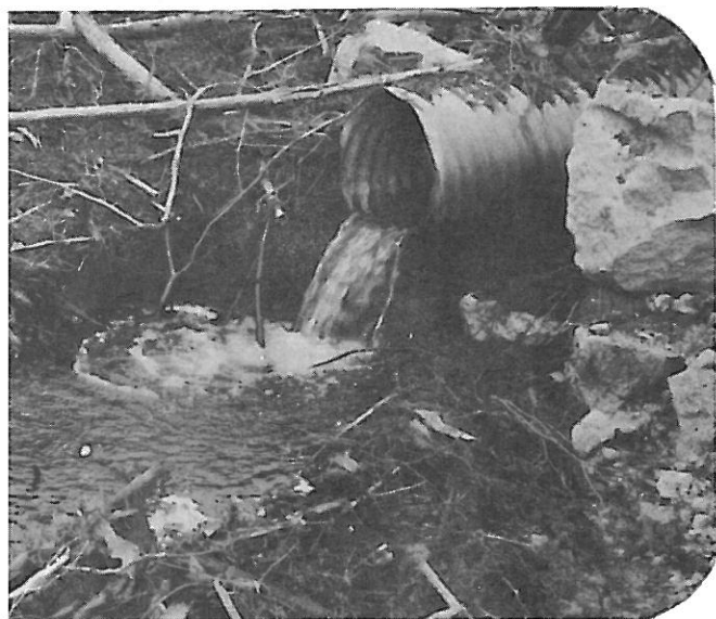
Figure 21.-- Small fish cannot pass through this culvert because of its elevation above the normal stream bed.
